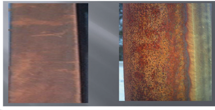
Surface Condition Aged Galvanized Steel Rating R-3 & R-4
